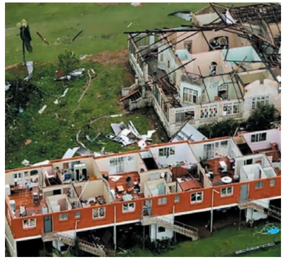
Figure 88: Houses and apartment blocks with their roofs blown off in Innisfail after Cyclone Larry struck in March 2006. Source: AP (Mark Baker)
