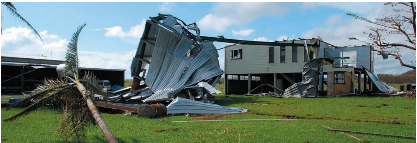
Figure 127: Very large wind-borne debris and the house it hit in TC Yasi.
