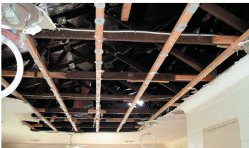
Figure 31: Collapse of ceiling from rain ingress via gable end during TC Larry. Source: CTS
