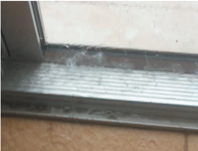
Rainwater bubbling through weep holes in windows.
