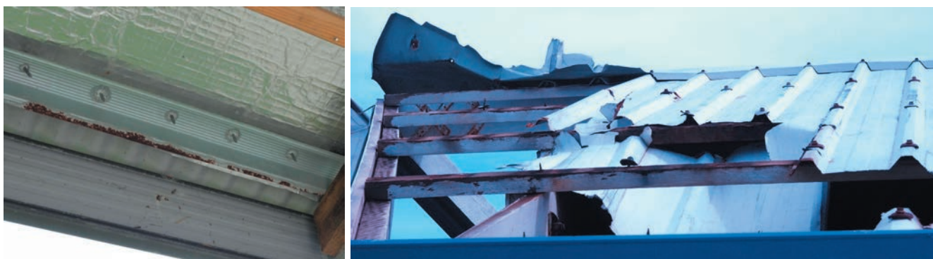
Figure 125: Examples of corroded battens and screws for properties near the coast. Source: CTS
