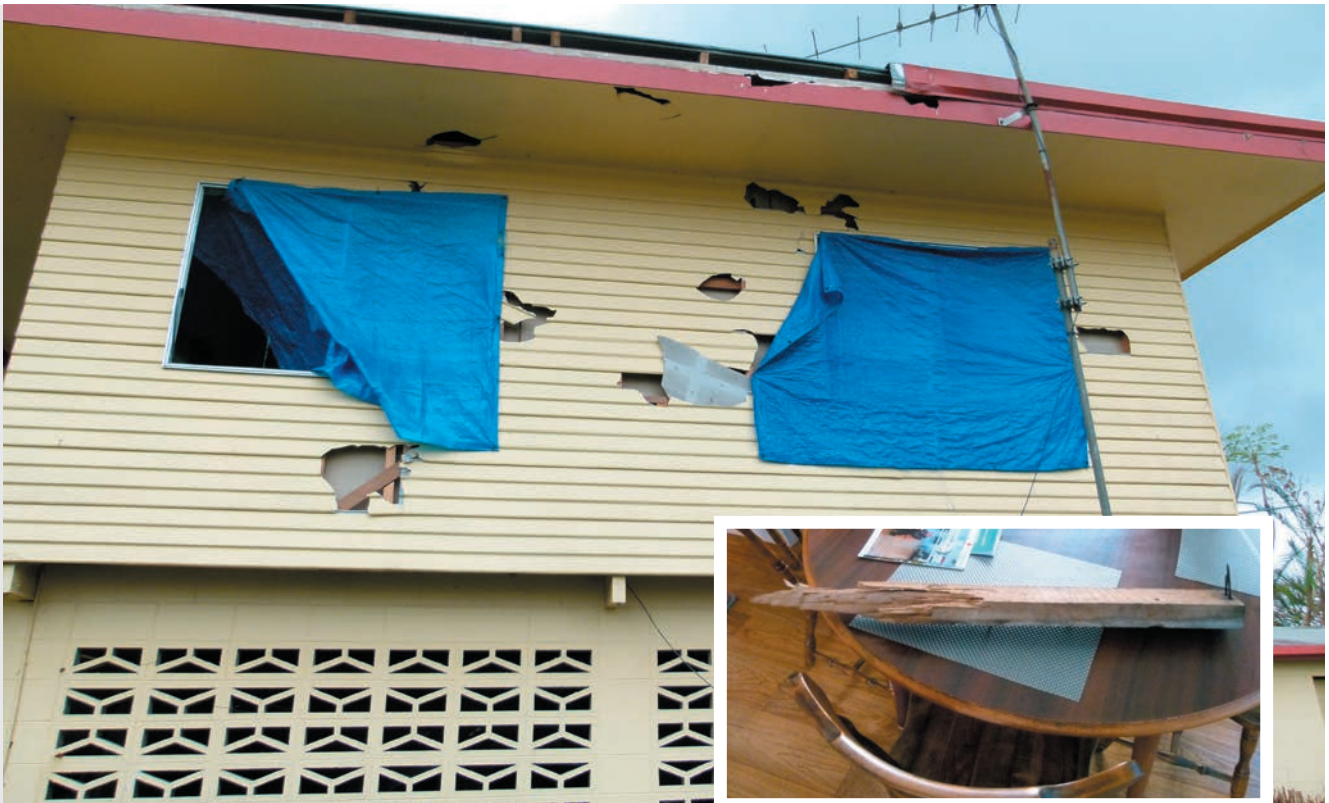
Figure 126: Complete penetration through window during TC Yasi (inset shows missile).
