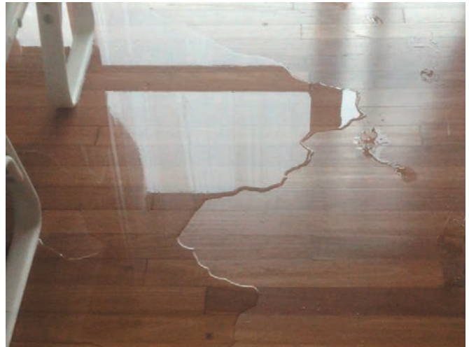
Water on timber floor.
