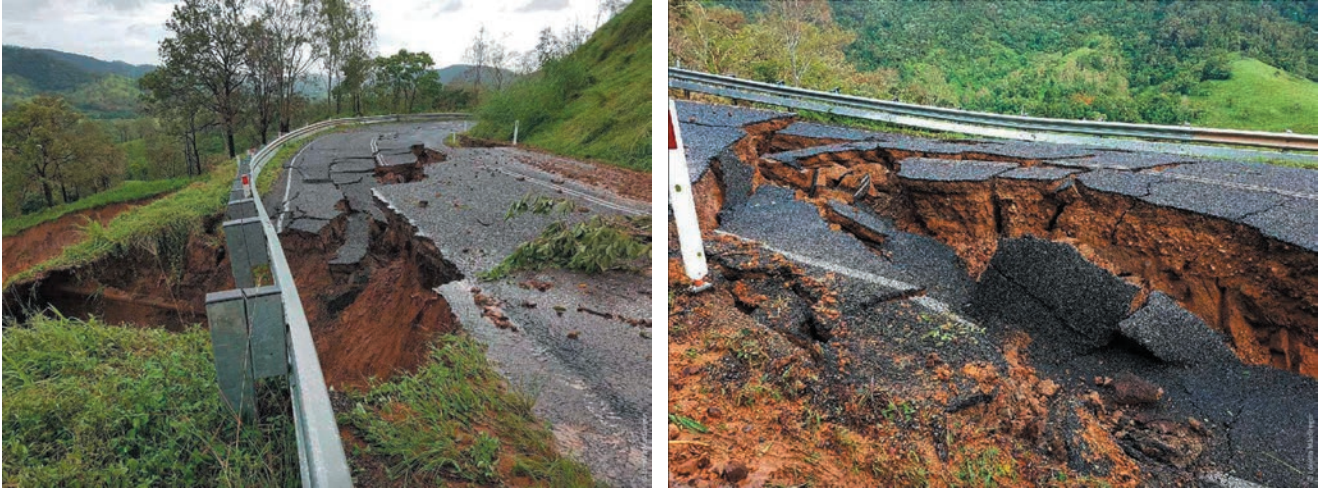
Figure 113: Serious damage around Sarina Range due to landslips from ex-TC Debbie. Source: Loretta MacGregor
