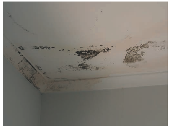
Mould on ceiling.
